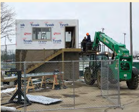
Crews have sectioned off part of the high school parking lot for construction of the new press boxes. Work is quickly wrapping up on the baseball, softball, and soccer press boxes before the Iowa winter sets in.
